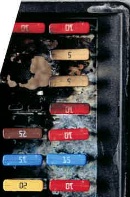
Damage to the circuit protective device when a non-standard fuse was used
